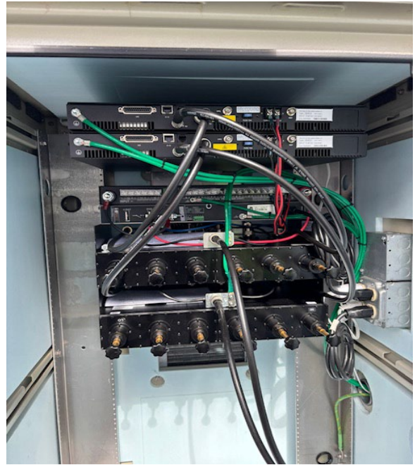
New Radio Repeaters for EMD & Highway Department in controlled environment cabinet
