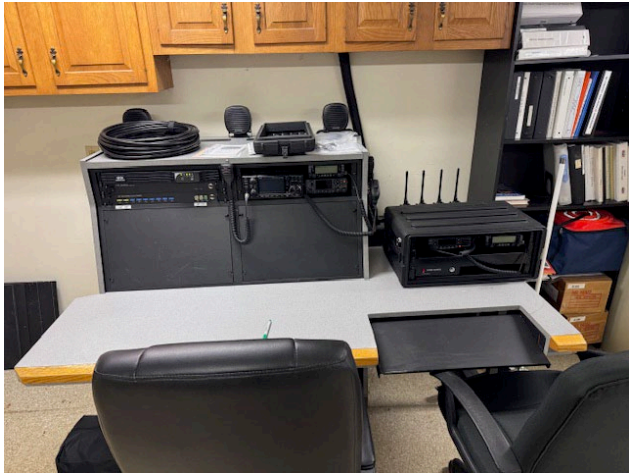
New TOC station for Emergency Communications
